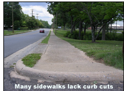
Many sidewalks lack curb cuts
